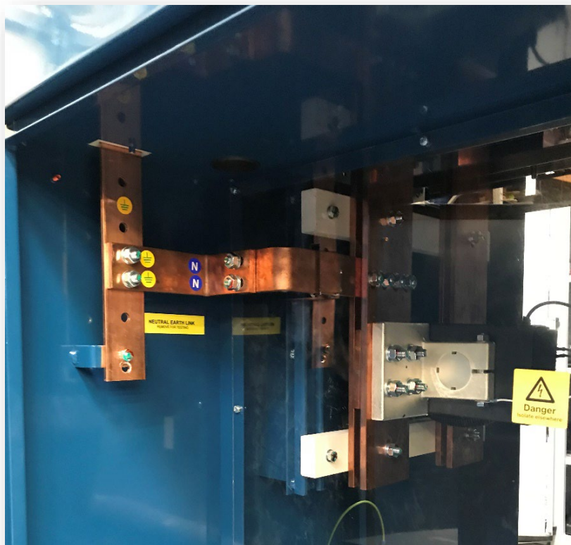
Figure 4 - Neutral - Earth link in a switchboard with thanks to of J.Peckham for permission to use the image
